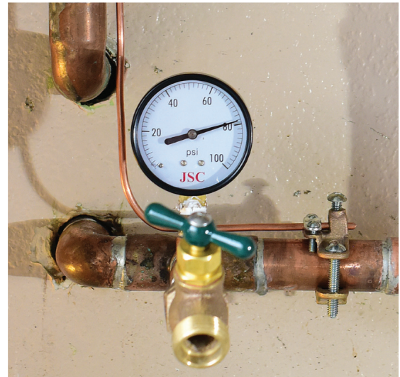
Figure 9 - Copper wire clamped to incoming water main
