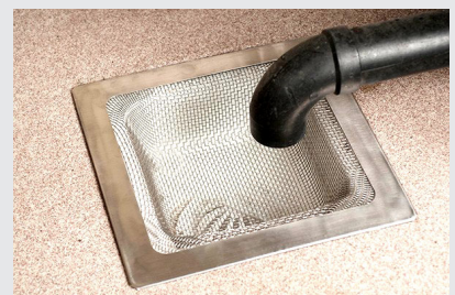
Figure 7 - Rinse line to drain.
